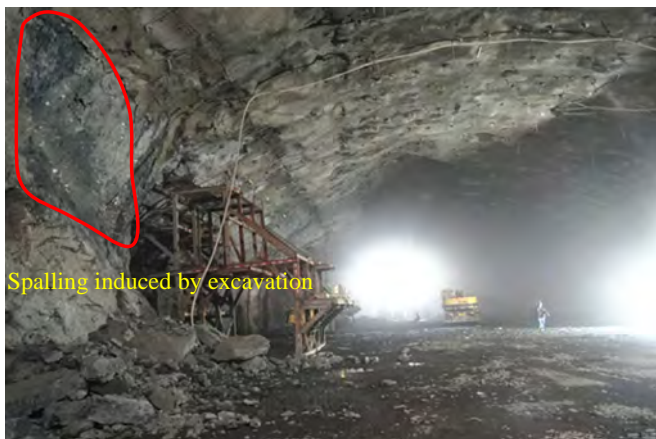
Fig. 5. Photograph of rock mass spalling in the main powerhouse.
