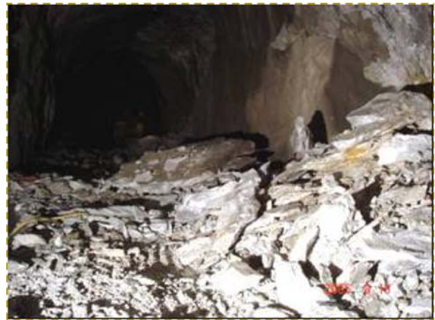
Fig. 10 Area of rock burst in the headrace tunnels of Jinping II
