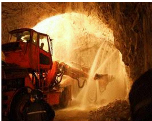
Fig. 11 High pressure ground water bursting in the access tunnels
