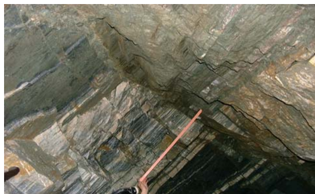
Fig. 14 Deep buried fissure in the left dam abutment of Jinping I
