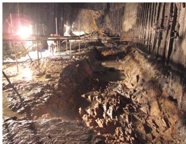
Fig. 13 Zone of crushed weak rock in the left dam abutment of Jinping I
